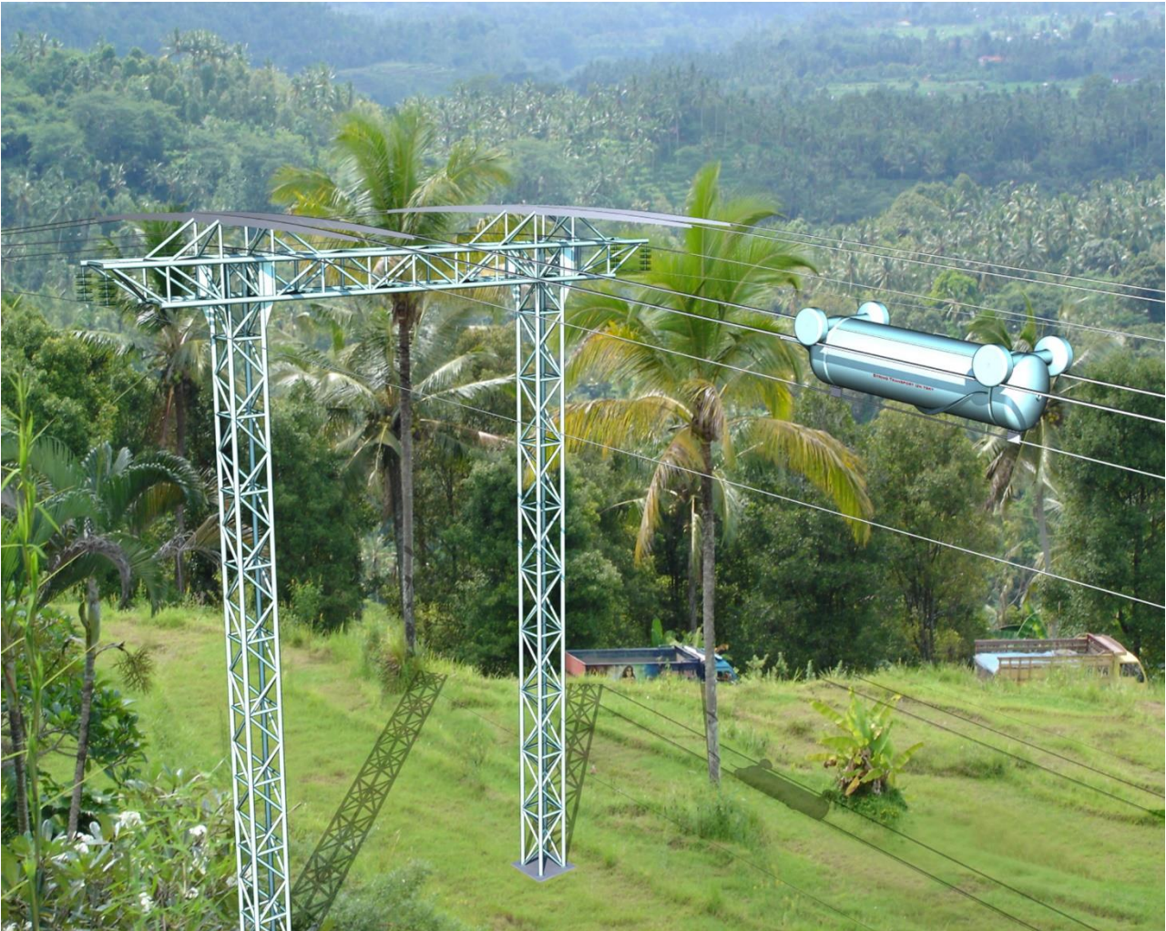
Fig. 7. Power and communication lines combined with container tracks
